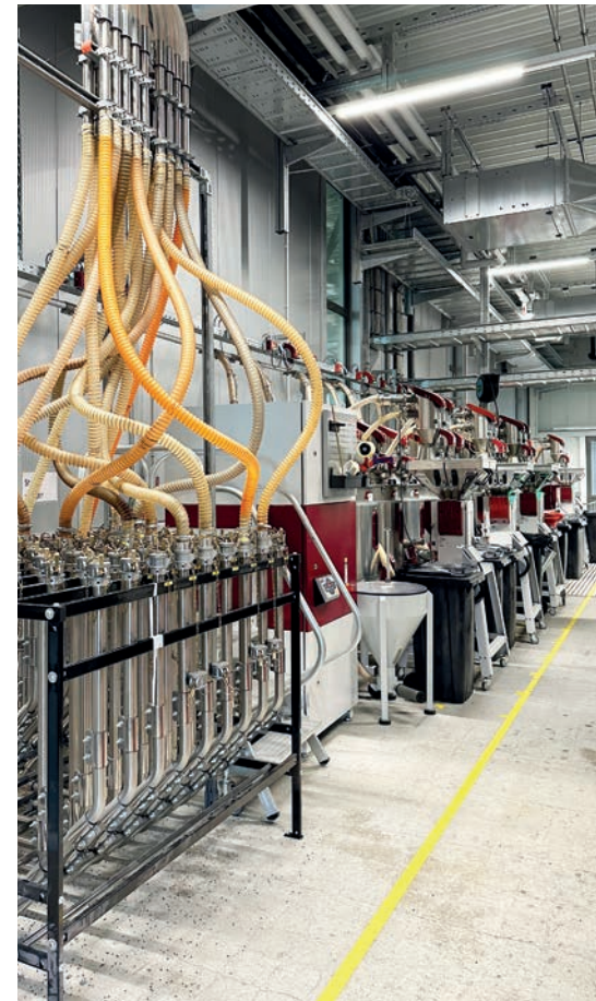
The granulate is fed into the materials handling system with gram-accurate precision by Gravimax gravimetric blenders from WITTMANN.
